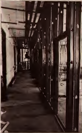
Labyrinth like ... Metal frames dividing the new offices were erected and will soon be covered by drywall.
